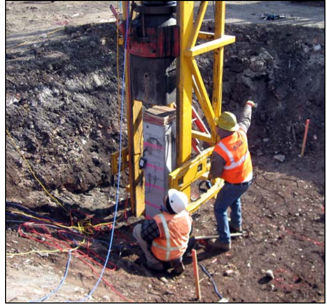
In this photo, the piling is being tested for in-bearing capacity. Each piling will be tested on the kcICON Project. The contractor, PCC, does Quality Assurance, and the owner, MoDOT, inspects the contractor's Quality Assurance process.
