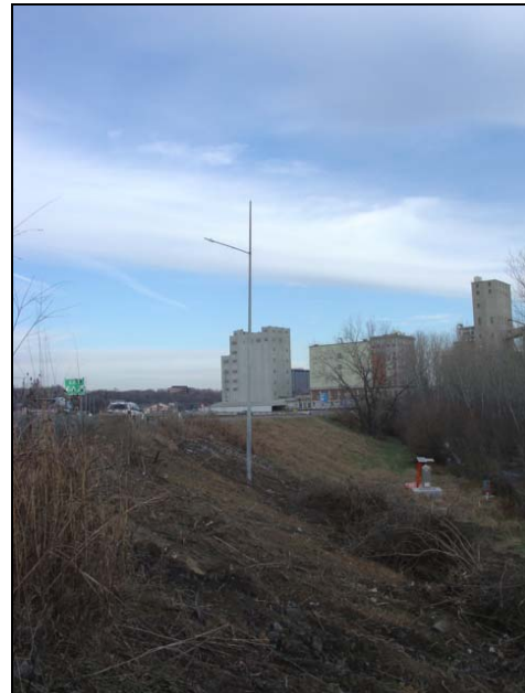
Top: A close view of the new LED light at the top of the Armour Rd. exit ramp. Bottom: The solar panels from the orange message sign used to power the LED light, are not visible to traveling motorists above.
