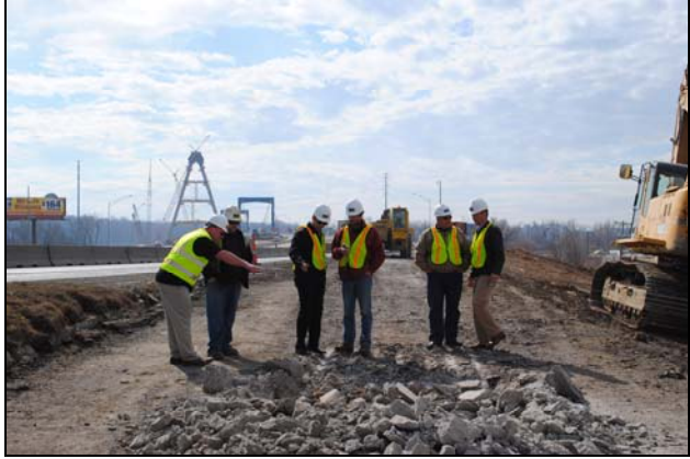
With the resonant machine in the background, RMI representatives and Czech Republic visitors inspect what was pavement, and is now rock fill on the kcICON Project.
