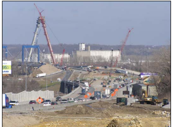
The Paseo ramp bridge demolition is complete. Excavation and grading work to construct the new interchange is under way.
