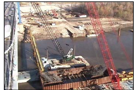
A view from the web camera that's positioned on top of the Paseo Bridge looking down into the cofferdam for the construction of the new bridge foundation.
